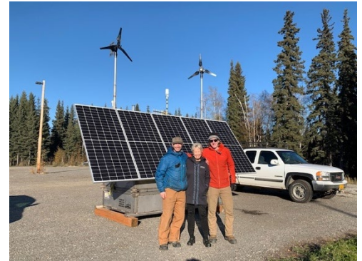
Molly McCammon, Hank Statscewich, and Jordy Maisch with the new remote power module lite to be used for High Frequency Radars in the Bering Strait.
