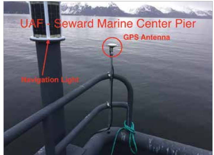
The AOOS/ASTRA GPS Antenna installation is located on the University of Alaska (UAF) – Seward Marine Center pier in downtown Seward, Alaska.
